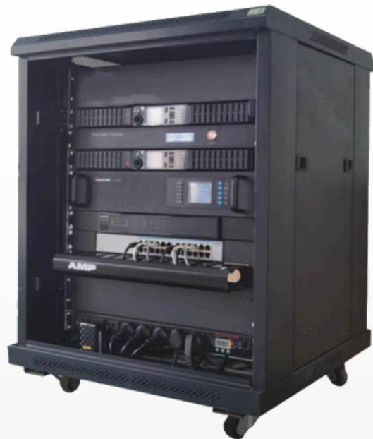
VHF Base Station
